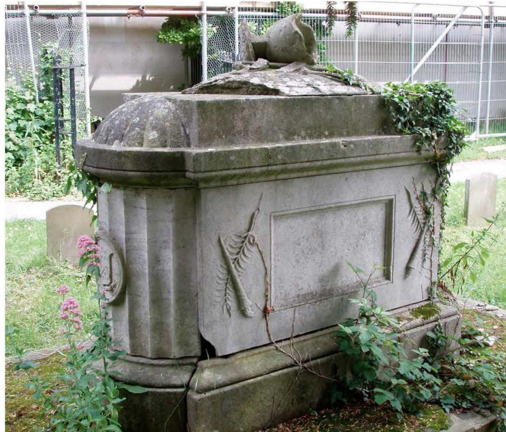
Figure 8 The Whyatt chest tomb in Egham churchyard, Surrey: notable examples of outdoor Georgian monuments will warrant listing. Listed Grade II.
